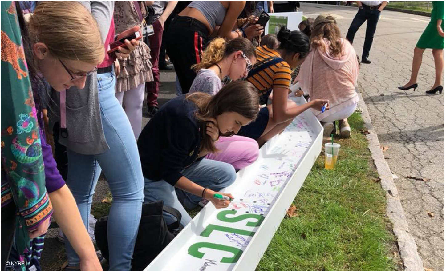
Sarah Lawrence Class of 2019 signs the steel beam before it is placed atop the new Barbara Walters Campus Center.
